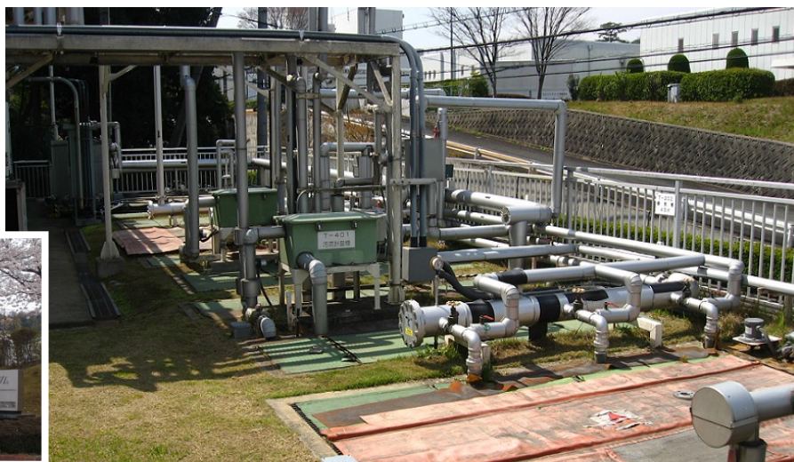
Overview of Wastewater Treatment Facility
