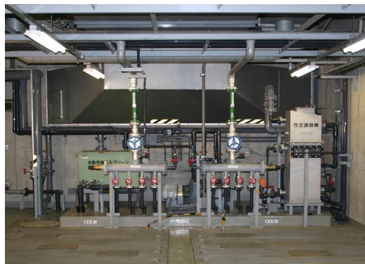
MBR facility overview
